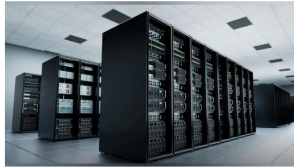
FIGURE 3. High-Density AI Compute with Integrated Cooling Infrastructure
